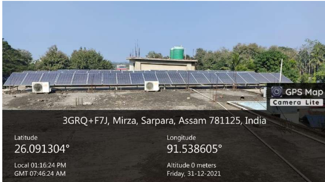
Fig. Installed Solar Panel
